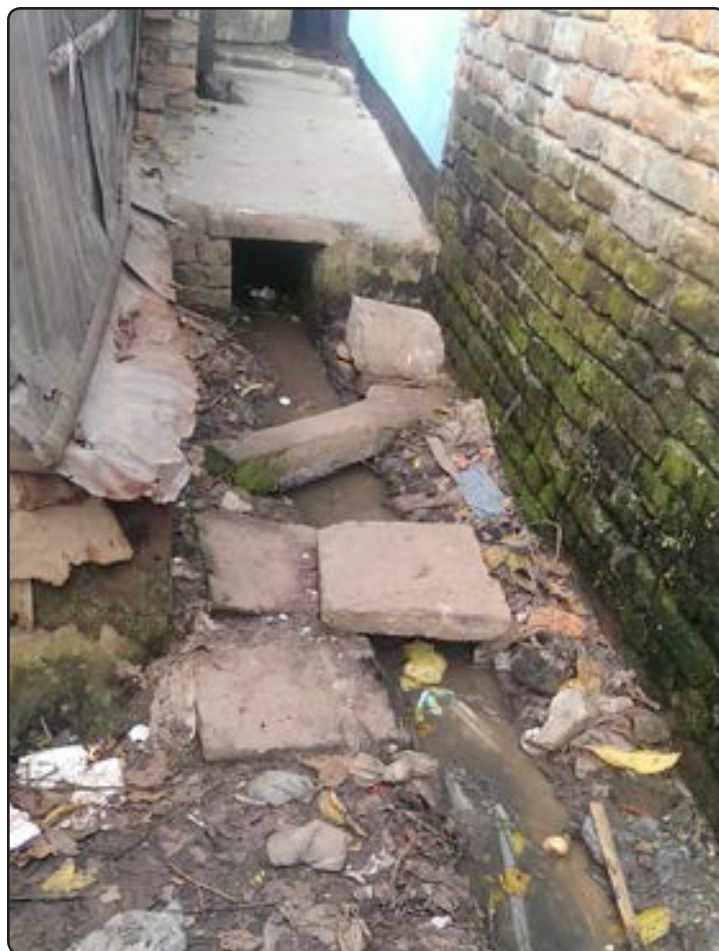
Fecal sludge being discharged into open environment.
