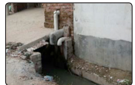
Household latrine directly connected to open drain.
